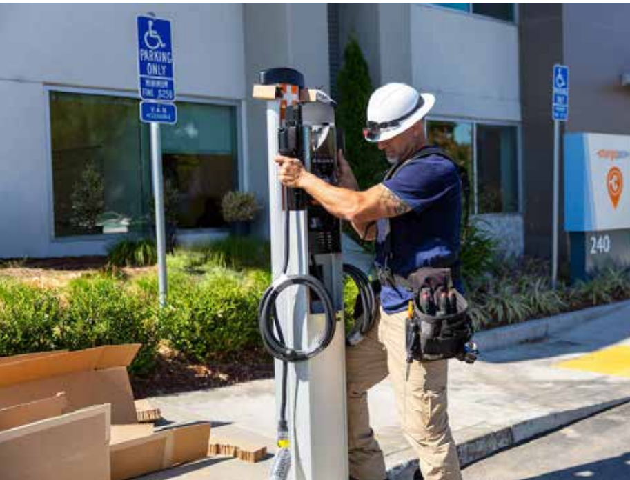
ChargePoint and the National Electrical Contractors Association are working together to develop training programs for electricians to teach them how to install EV charging infrastructure.
